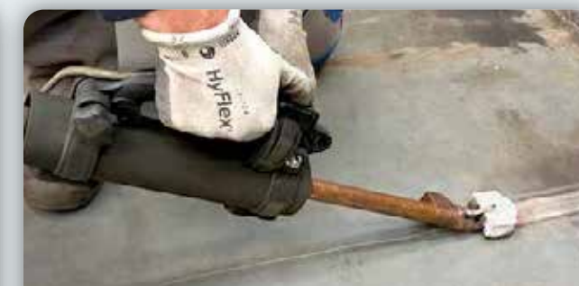
SHIPYARD - CONSTRUCTION NAVALE Inductor L20/B4 Powerduction 220LG
